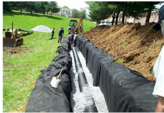
Infiltration trench Chester County, PA
