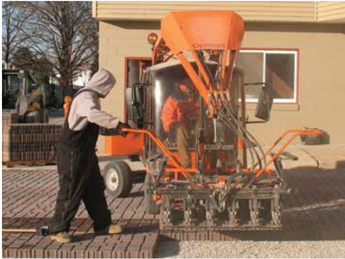
Installation of porous pavers at the Energy Exchange in Milwaukee, WI (November 2009).
