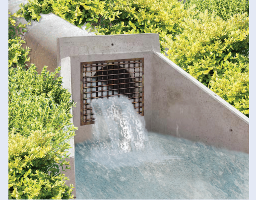
Storm sewer pipes in good repair can handle larger volumes of water runoff.
