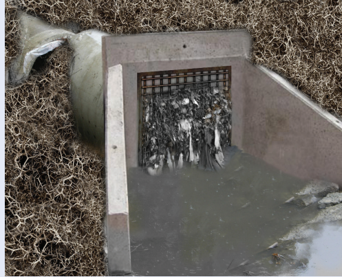
Storm sewer pipes are clogged or corroded, so they handle less water runoff.
