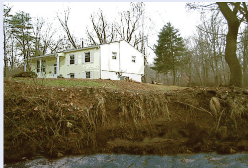
Eroding streambanks fill streams with mud, and these streams flood more quickly.
