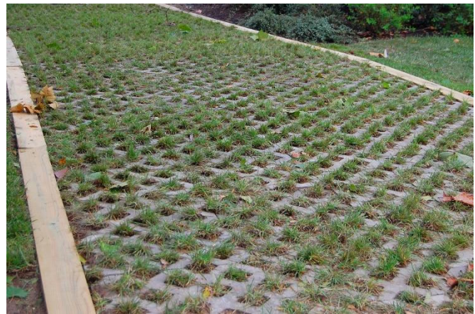
Figure D-1-2. Permeable pavement is a type of runoff reduction (RR) practice because it allows processes such as filtration and evapo-transpiration to occur. This approach reduces runoff and removes a greater portion of pollutants than stormwater treatment (ST) practices that employ a permanent pool – such as wet ponds, wet swales, and constructed wetlands – because such practices simply provide storage and treatment before discharge. Photo: Chesapeake Bay Program
